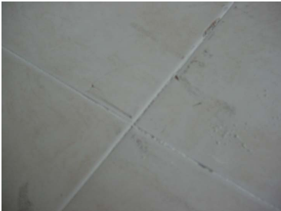
Figure 5-4: Some cracking of the tiles on the concrete plinth was evident after a number of tapping tests. The tapping machine position was adjusted to not impact upon the fracture lines for subsequent tests. We do not consider the small amount of cracking to significantly affect the measurement results.
